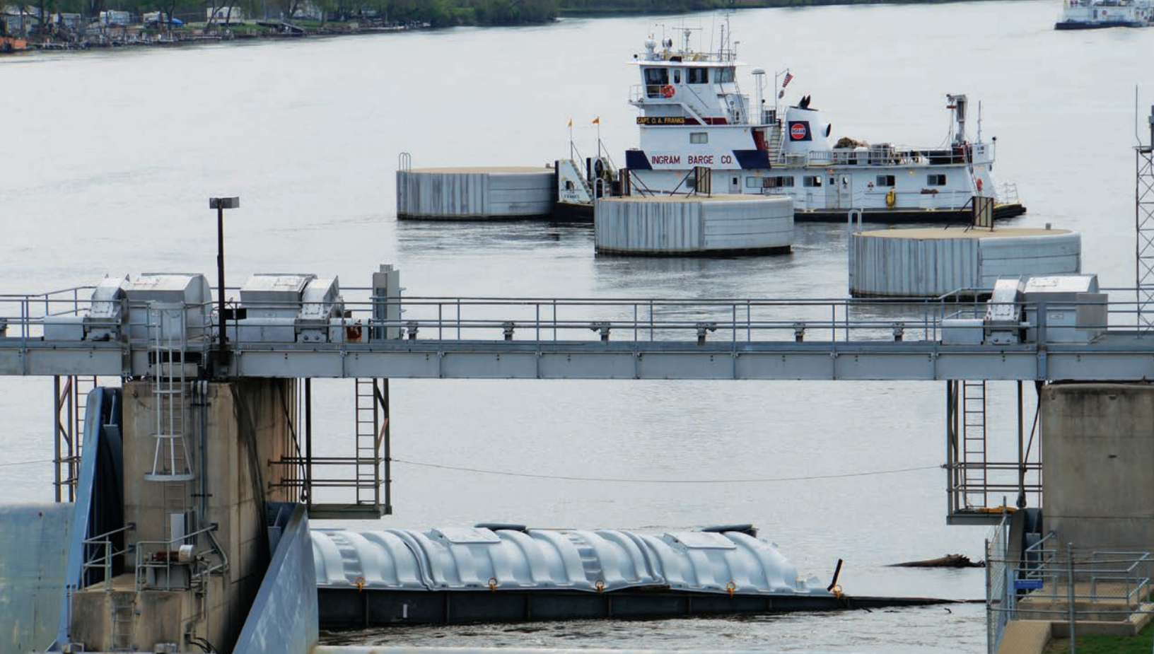
FIGURE 23.6 A partially sunken barge in April of 2013 blocked the flow of floodwaters and damaged the Tainter gates that control the level of water in the pool behind the Marseilles Dam.
