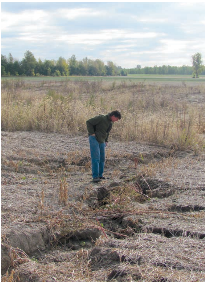
FIGURE 13.6 Rill and gully erosion occurred after planting soybean in 2013 on regraded slopes and filled land.
