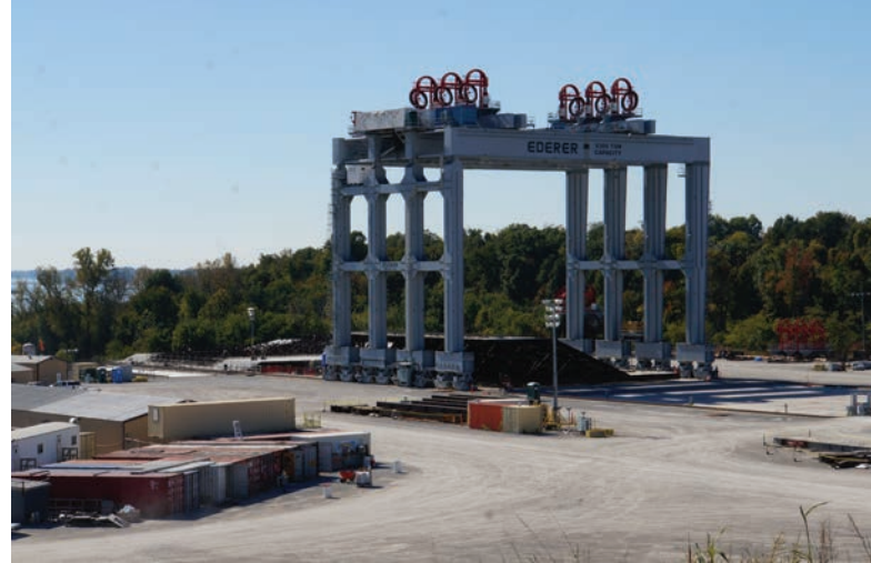
FIGURE 18.9 A giant 5,304-ton lift built on the construction site of the Olmsted Lock and Dam is used to carry cement frames to barges on the Ohio River for placement in the river.
