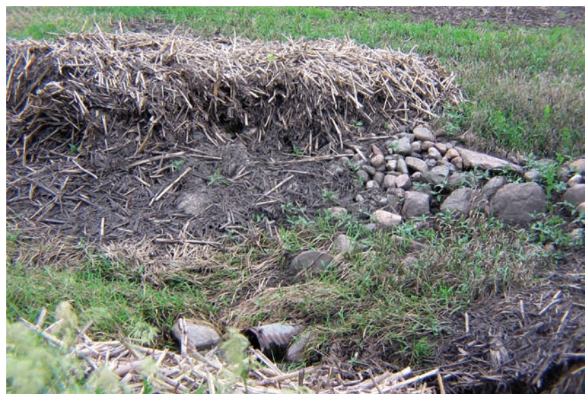
FIGURE 9.8 Corn stalks clog drainageways, waterways, and culverts after flood events.
