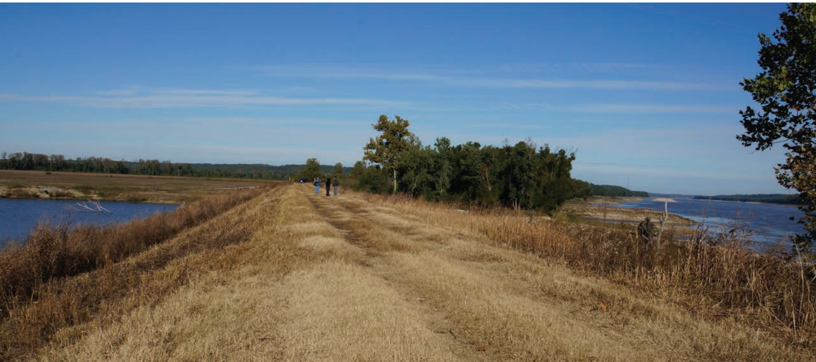
FIGURE 7.4 The Commerce Farmer Levee and Drainage District repaired a 2011 levee breach located two miles south of Commerce, Missouri. Note the Mississippi River on the right and the crater lake on the left created by the force of water pouring through the breach.
