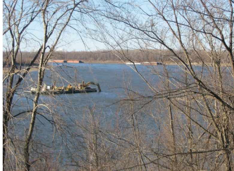
FIGURE 22.2 River bottom bedrock is dredged using an excavator to increase the navigation depth.
