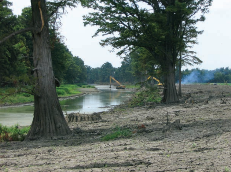
FIGURE 11.7 Two excavators remove sediment from a drainage ditch and spread it on the stream bank surface.
