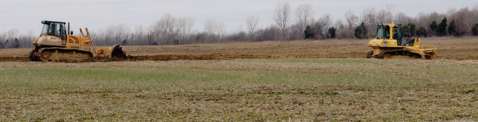
FIGURE 8.9 Bulldozers push soil into wetlands and ponds at the bottom of the gullies in O'Bryan Ridge.
