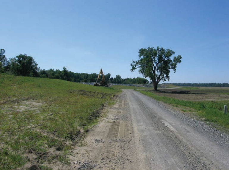
FIGURE 11.3 The site of the third explosion on the frontline levee is located near Big Oak Tree State Park. The levee is being reconstructed where the crater lake extended into agriculture lands.
