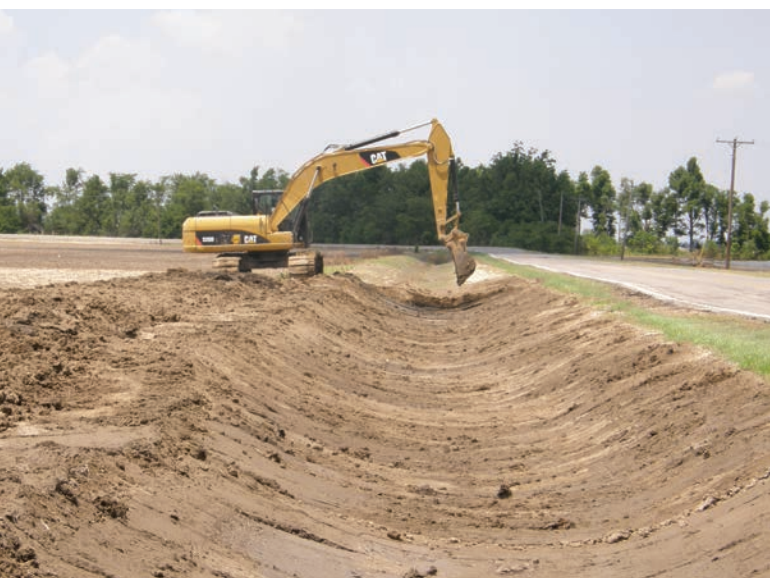
FIGURE 10.2 Excavator cleaning out sediment in road ditches. Photo credit: Brett Miller, USDA Natural Resources Conservation Service soil conservation technician.
