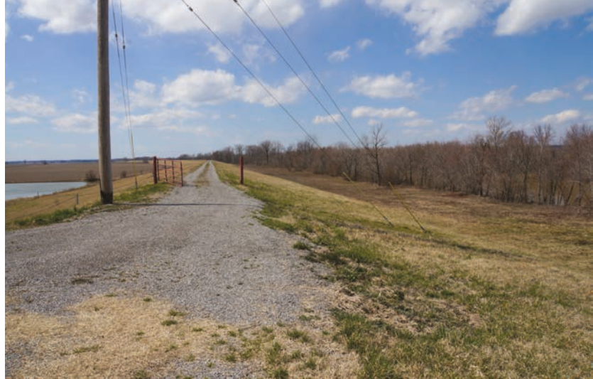
FIGURE 5.5 The diversion embankment protects agricultural bottomlands from the Missouri Ozarks upland stream runoff and Mississippi River backwater at flood stage.
