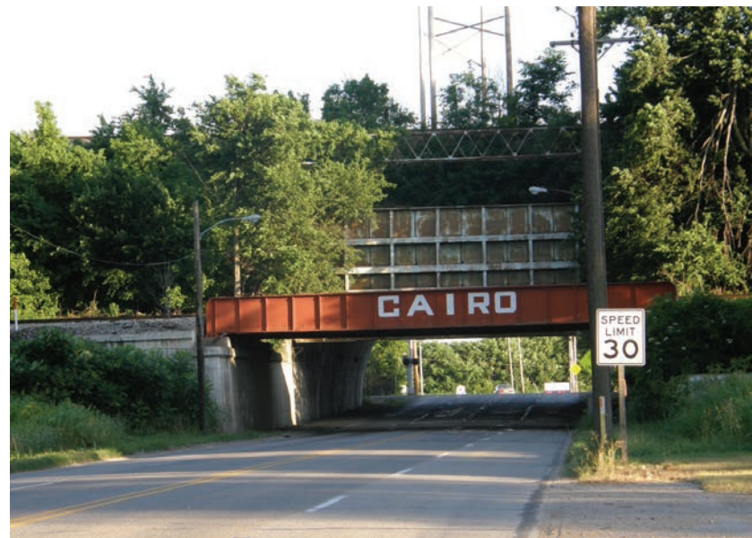
FIGURE 16.4 A walled city. A raised railroad bed serves as a levee for the northern boundary of Cairo, Illinois, and provides an entry to the levee-enclosed city for Illinois Route 3 traffic. Flood gates on this entry could seal the city behind embankments and the floodwall if levees north of the city were to fail.
