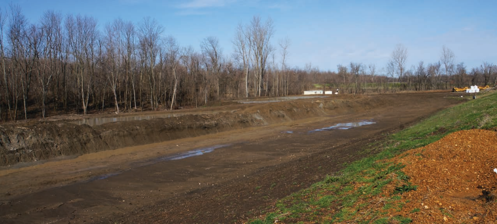
FIGURE 17.8 This slurry trench between the levee and Mississippi River creates an impervious barrier that reduces river pressure and seepage.
