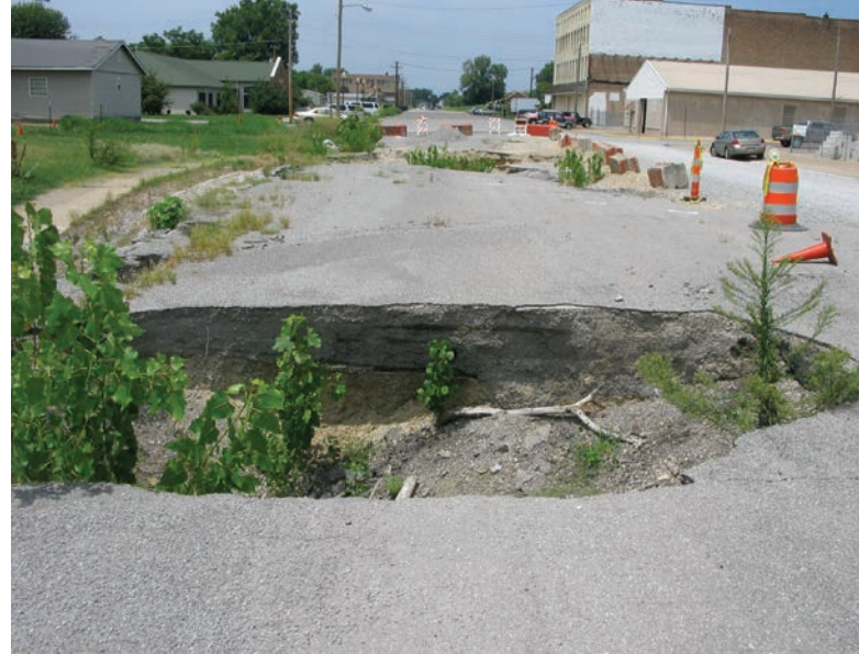
FIGURE 17.1 The Commercial Avenue sinkholes in Cairo were near or above the sanitary sewer lines.
