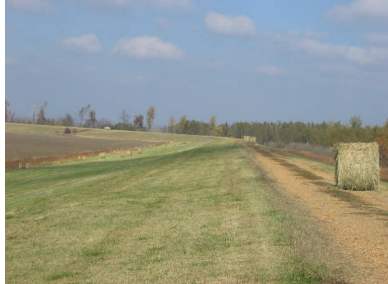
FIGURE 15.3 Routine management of vegetation on the Commerce to Birds Point mainline US Army Corps of Engineers levee protects against woody encroachment and tree roots that can undermine the strength of levee structures.
