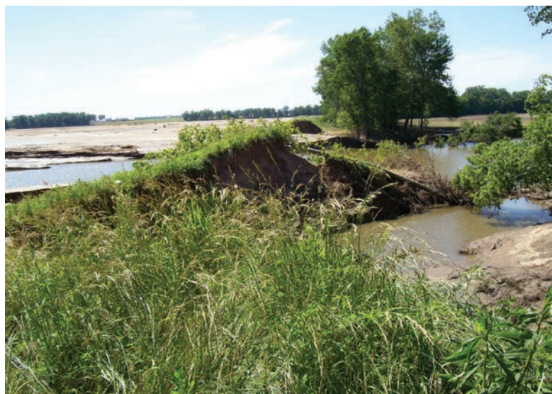
FIGURE 9.4 The Embarras River cuts through a levee near Sainte Marie, Illinois, in June of 2008.
