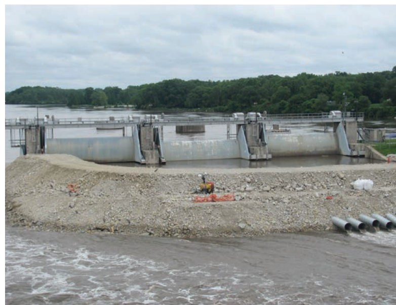
FIGURE 23.10 The US Army Corps of Engineers constructed a dike and pond to temporarily manage the water pool behind the dam after the gates were damaged in April of 2013 at Marseilles.
