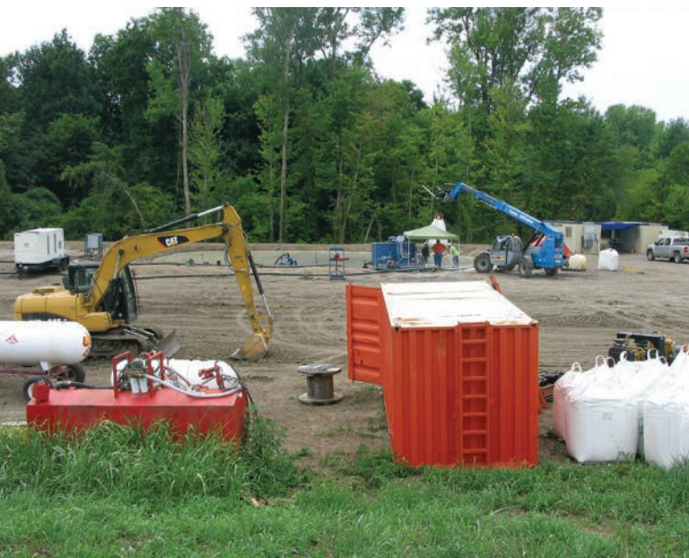
FIGURE 17.7 Bentonite bags are dumped into these slurry ponds and mixed with water to create slurry for the trench.
