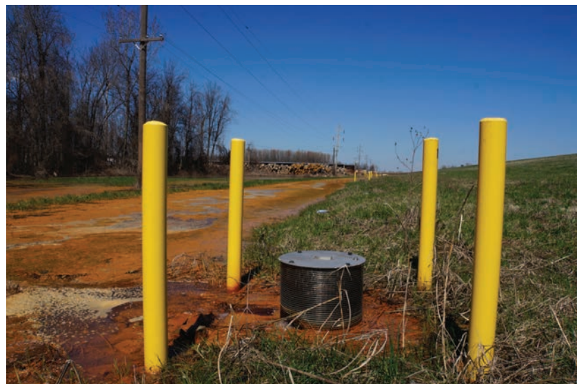
FIGURE 17.5 A series of relief wells pump iron-rich, yellowish-red groundwater into a drainage ditch to relieve substratum pressure when the river is higher than the land inside the levee. The water is collected and pumped over the levee.
