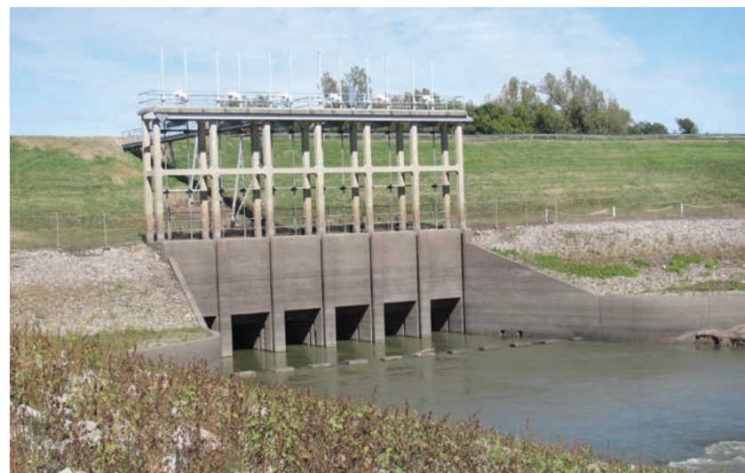
FIGURE 7.2 When open, the New Madrid Floodway setback levee gate drains the 200,000-acre St. Johns Bayou basin to Main Ditch and into the Mississippi River. It is closed under flood conditions to prevent Mississippi River backup water from flowing into the basin.
