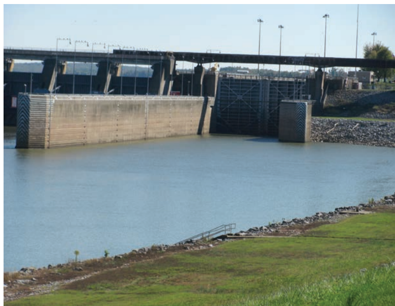
FIGURE 20.2 A railroad built above the Barkley Lock and Dam on the Cumberland River transports iron ore and manufactured products.
