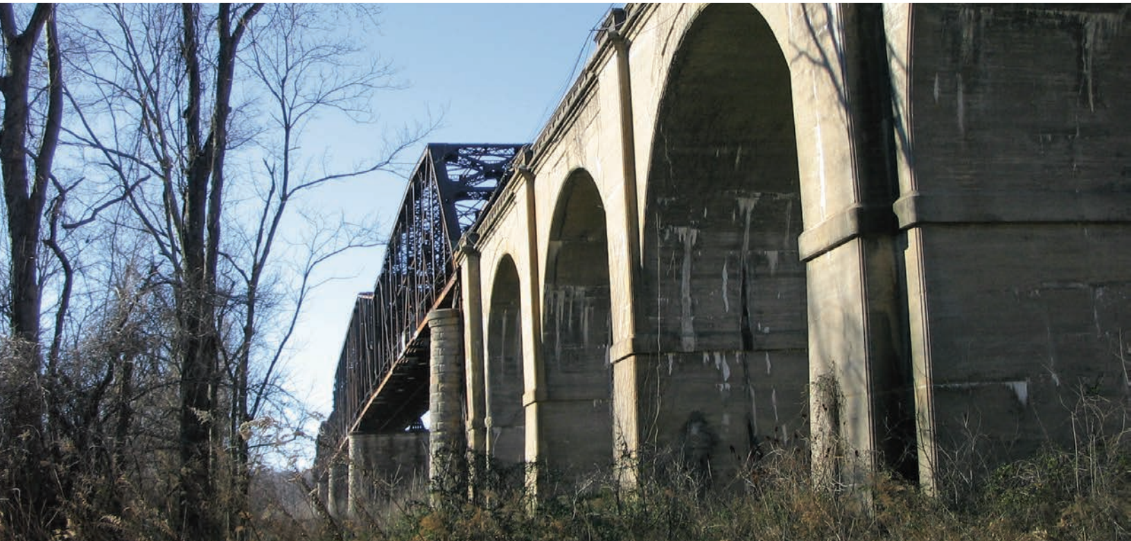
FIGURE 22.4 The reinforced concrete, two-track railroad bridge was built in 1905 to connect Illinois to Missouri and enabled east-west commerce throughout the region.
